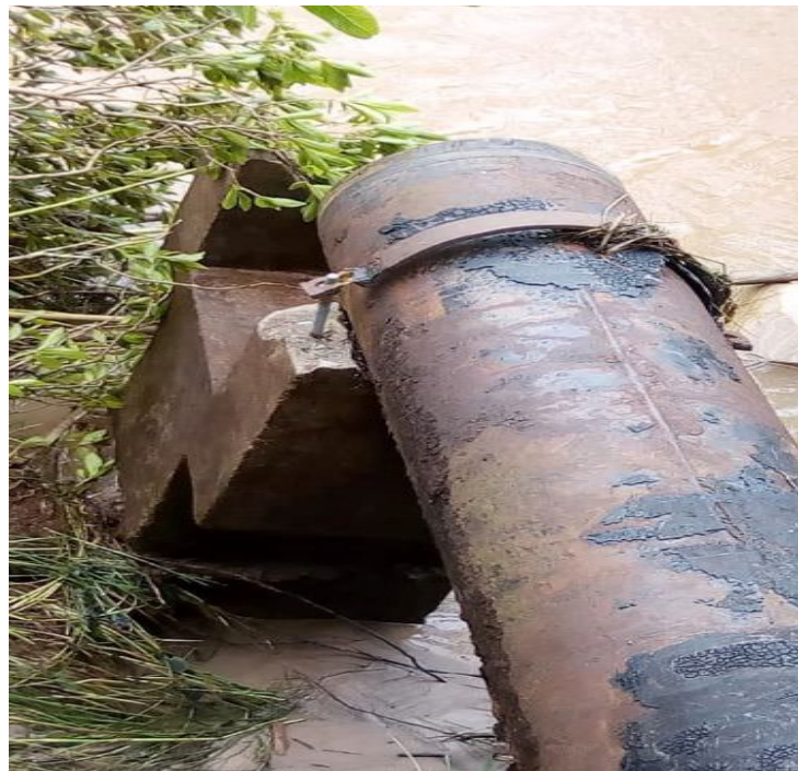
Figure 6: Water pipeline from Council's main source washed away after heavy rainfall
