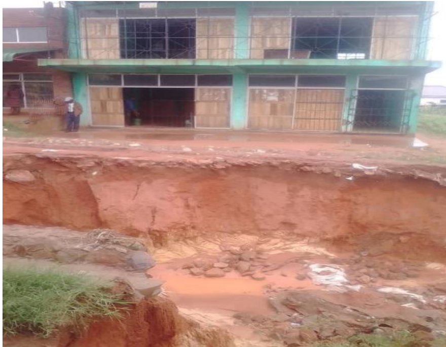
Figure 2: Damages caused by Cyclone Idai in 2019 in the Chipinge Town CBD
