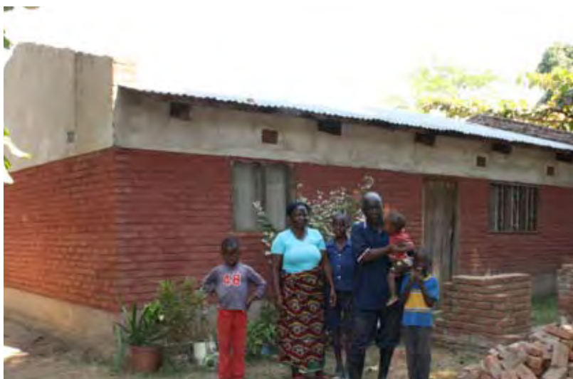
Photo: UN-Habitat - Surveyed Retrofitted House: Karonga / S 09°56'46.96" - E 033°56'5.68" 1 SHELTER PROJECTS 2010 - UN-Habitat / UNHCR / IFRC;
