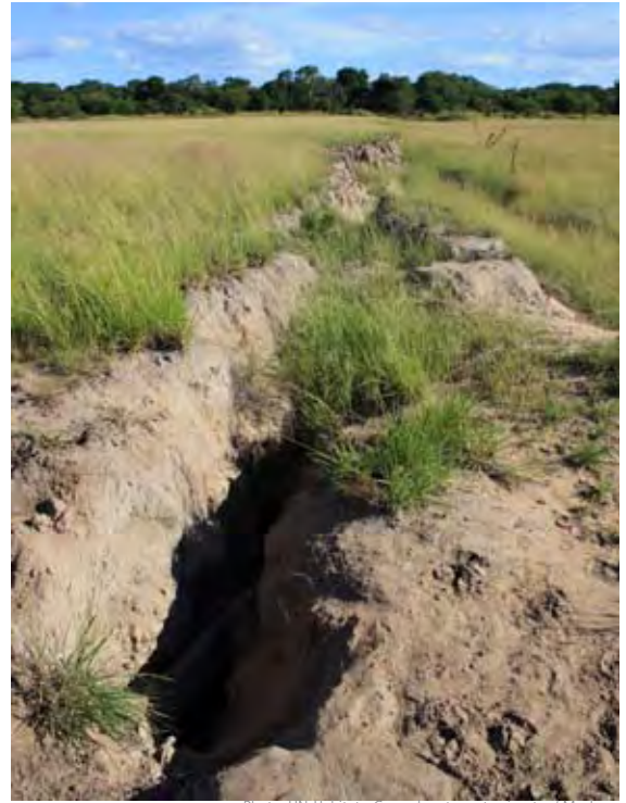
Photo: UN-Habitat - Ground rupture at epicentre / Machaze
