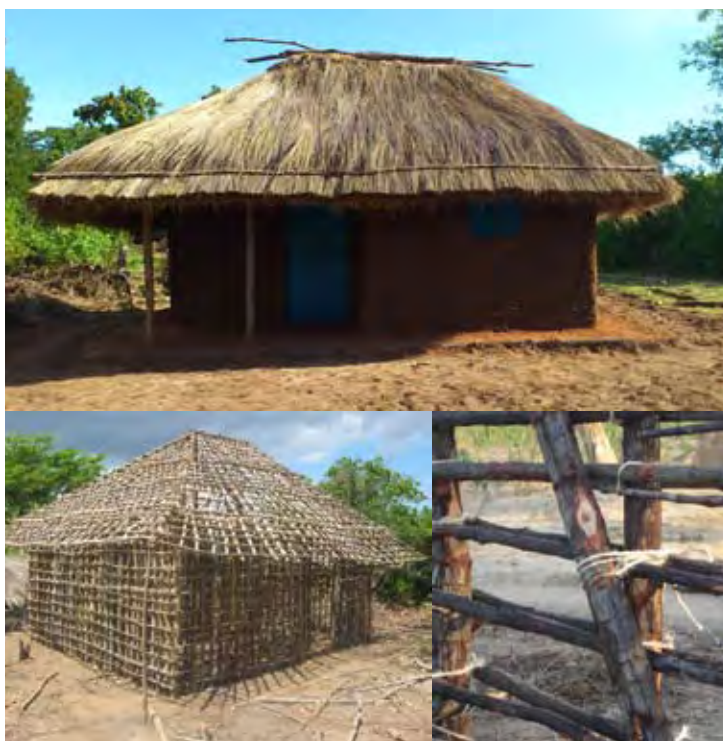
Photo: UN-Habitat - Reinforced Houses made in wooden sticks framework with improved anchorages
