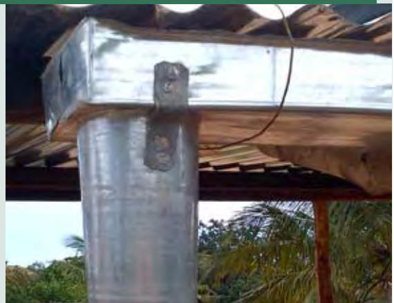
Photo: IRD - Water tanks / Mabiñale, Massinga District
