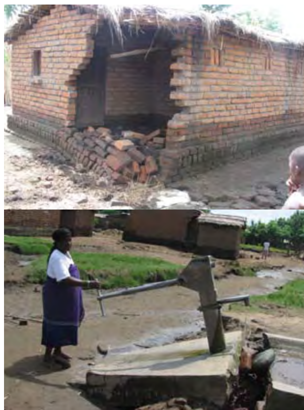
Photo: UN-Habitat - Houses and Community Infrastructures damaged by the floods
