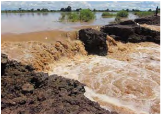
Photo: 2009 Karonga Earthquake damaged dyke lets in flood water / DoDMA
